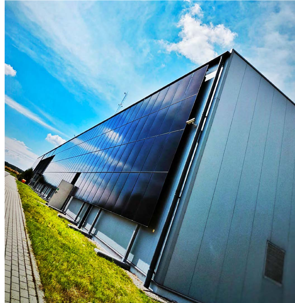
Solar panels on the facade of one of our factory buildings in Poland.
